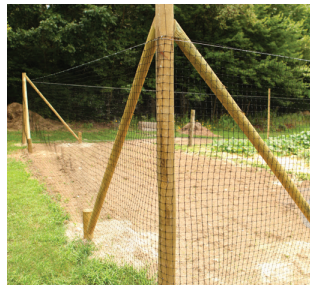
Above: 91" high Tenax is a quick and effective exclusion fence for light deer pressure. Can be used in conjunction with an electric offset.
